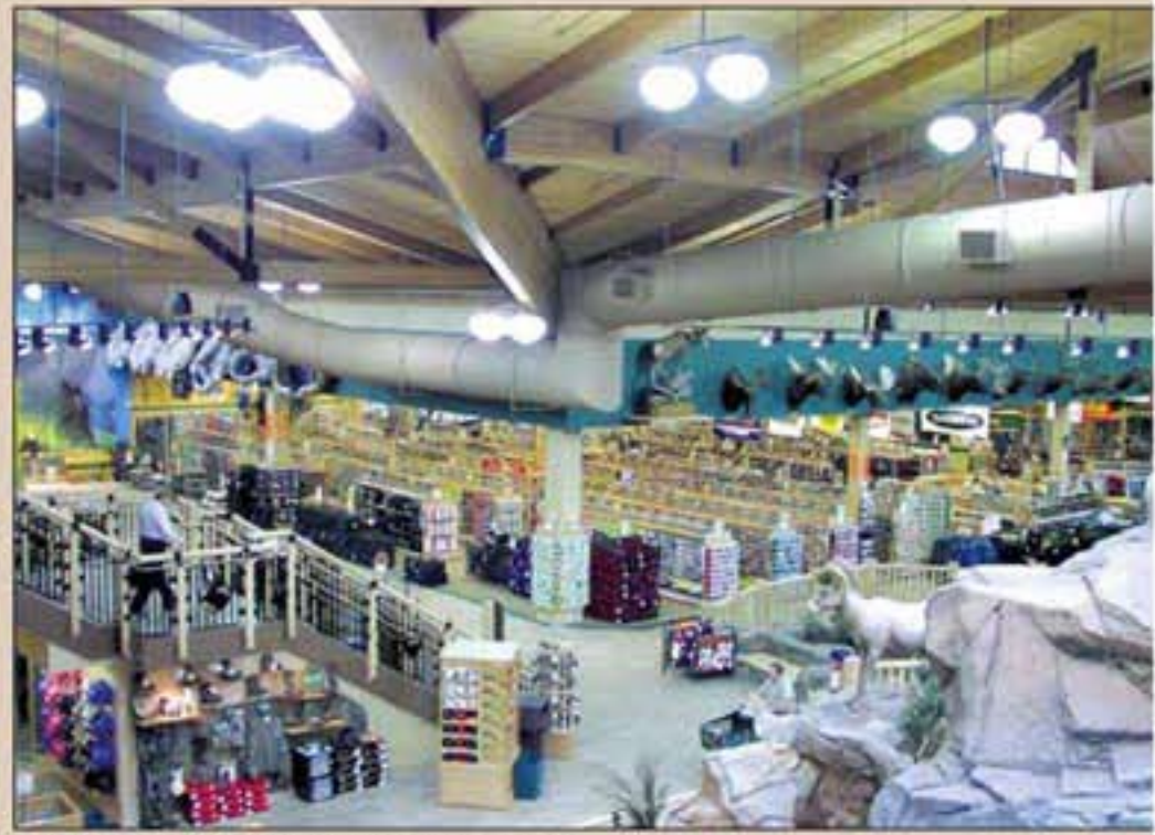
The ductwork hangs far above the store below.
