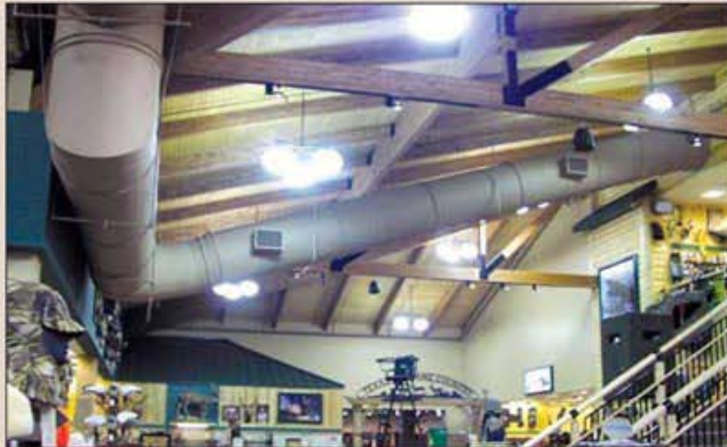
The spiral ductwork mounted in the Fort Worth, Texas, store. The taps were shop-mounted parallel to the floor at a 17 1/2- and 5 1/2-degree roof pitches.
